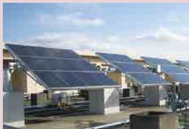
▲ Single-axis tracking type photovoltaic cell
