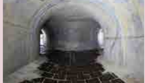
▲Pump well connection
