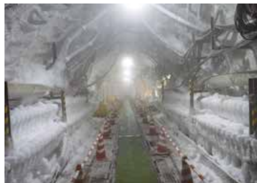
Fig.11 Inside the pipe in freezing
